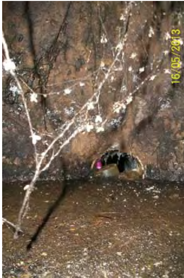
Plastics causing blockages in pipe work
