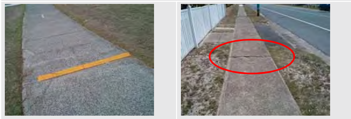
Tripping hazard on Marine Parade shared use path
