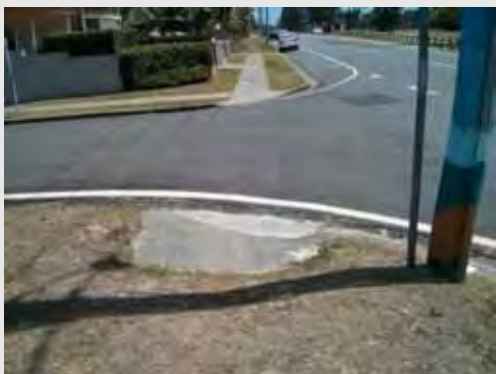
Disjointed footpath north of Beach Street
