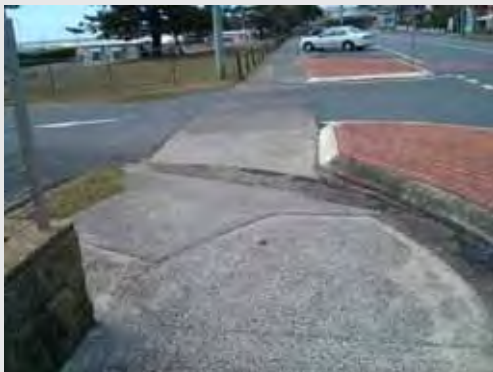
Steep kerb ramp at Bowls Club entrance, Kingscliff
