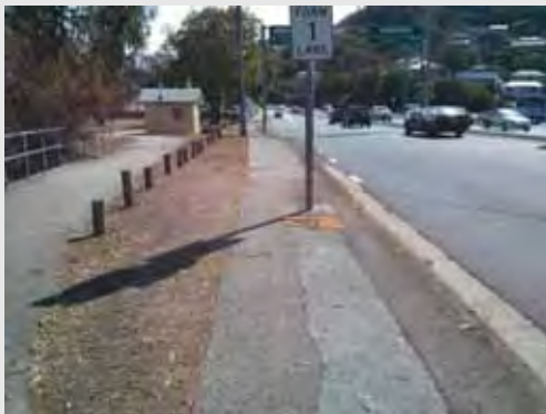
Sign pole obstructing footpath on Wharf Street
