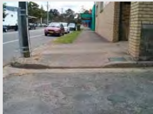
Tripping hazard on kerb ramp at Holstons Lane, Murwillumbah
