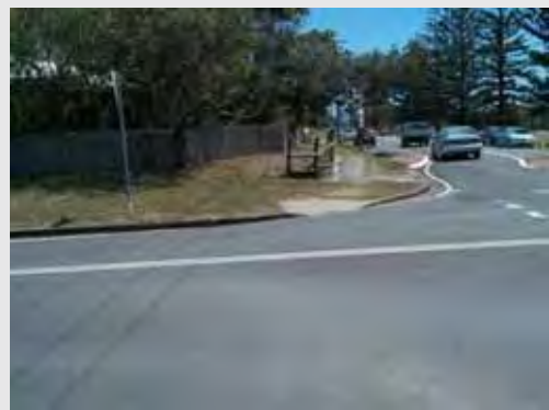
Disjointed footpath north of Ozone Street
