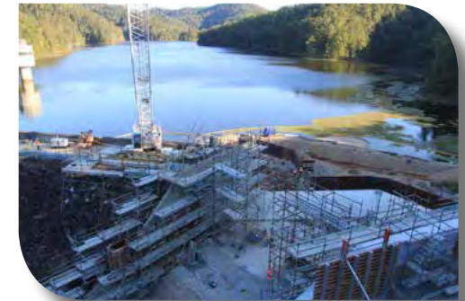
A $7.3 million major upgrade to Clarrie Hall Dam was delivered on schedule and under budget.
