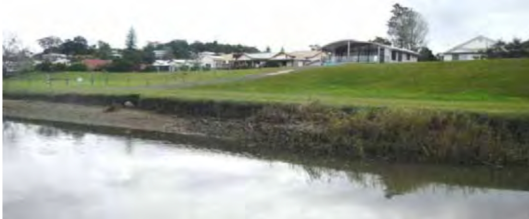
Photo 113 – showing minor erosion along bank toe
