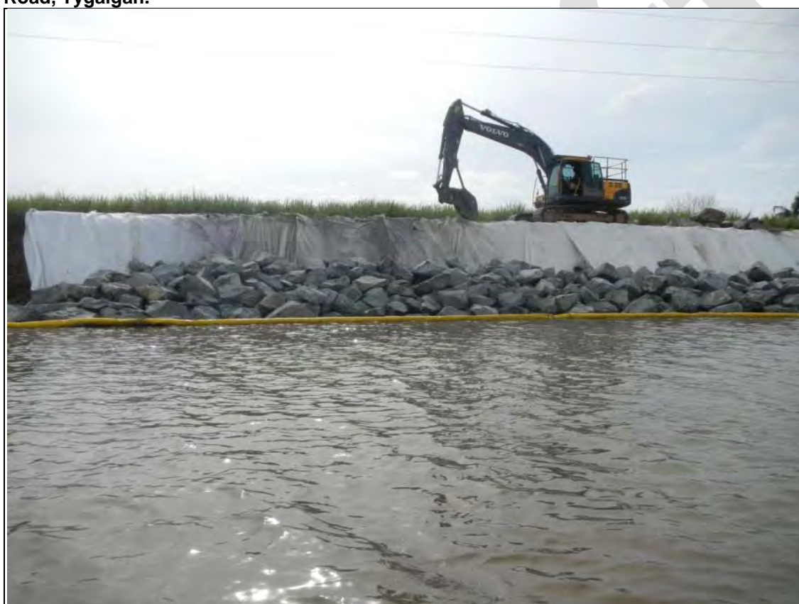
Figure 2. Reactive riverbank erosion stabilisation works being constructed adjacent to Tumbulgum Road, Tyngalga.
