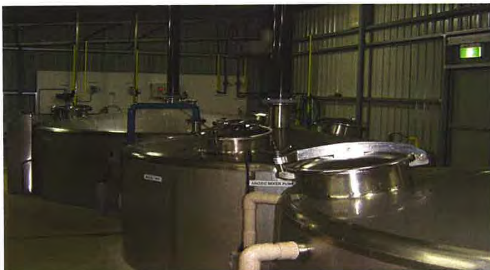
Figure 5-2: Photo of existing MBR treatment works at Forest Resort (Creswick, VIC)
