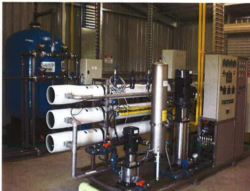
Figure 5-4: Reverse Osmosis unit with comparable capacity to RO1 at (Bridge Water Vic).
