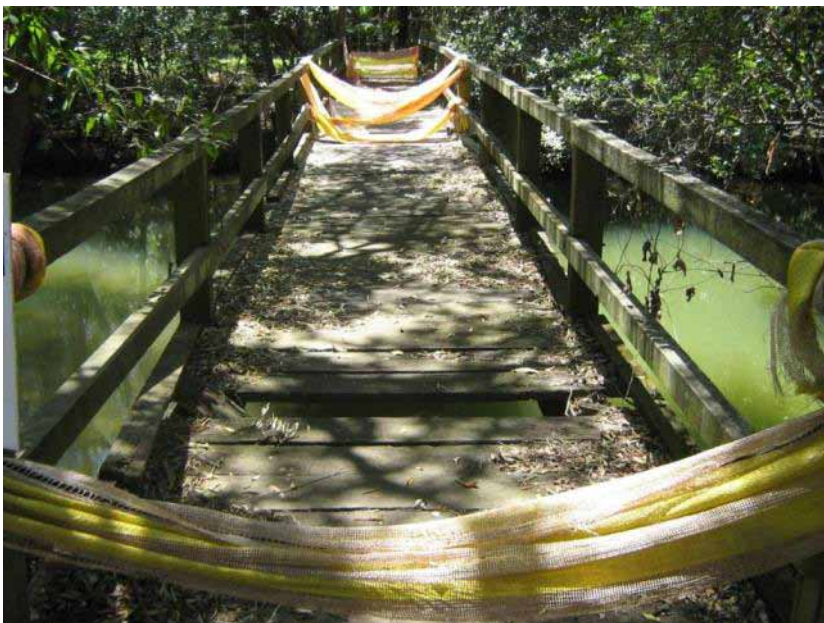
Photos 4 and 5: Dilapidated bridge
