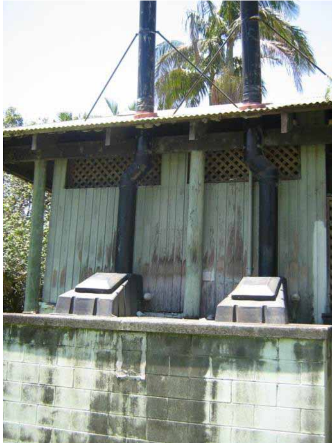
Photo 1: non-functioning wet compost toilets
