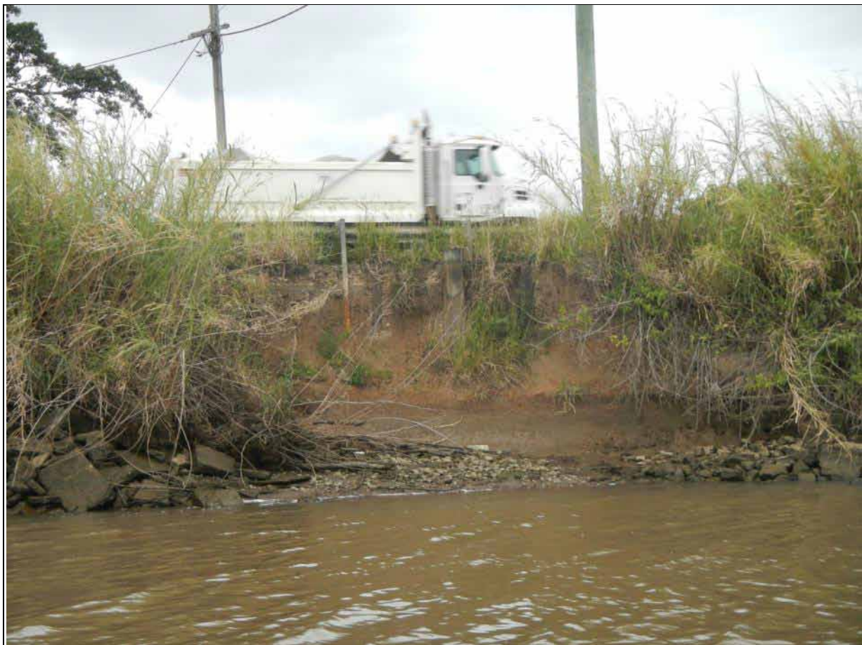
Figure 3. Bank slip adjacent to the Tweed Valley Way near Stotts Island. Road safety barrier anchor posts can be seen exposed in the top of the bank.
