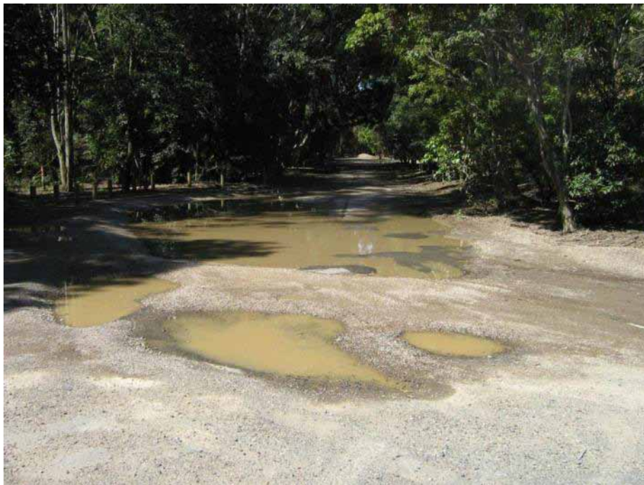
Photo 6: section of access road subject to regular inundation.
