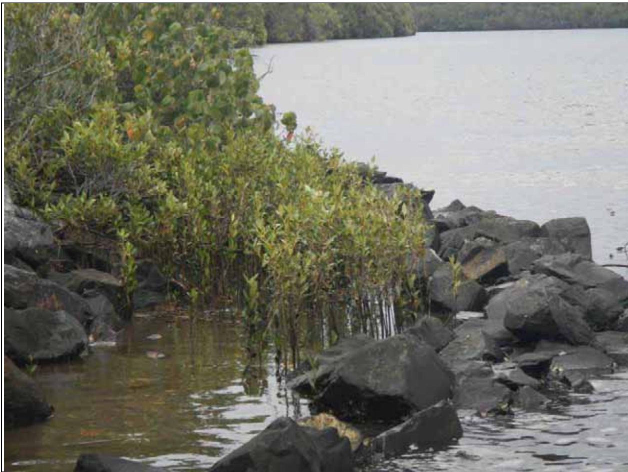
Figure 2. Rock fillets constructed on Chinderah bay drive showing natural mangrove recruitment. This area provides excellent fish habitat, a high level of erosion protection and will eventually have a very low visual impact.
