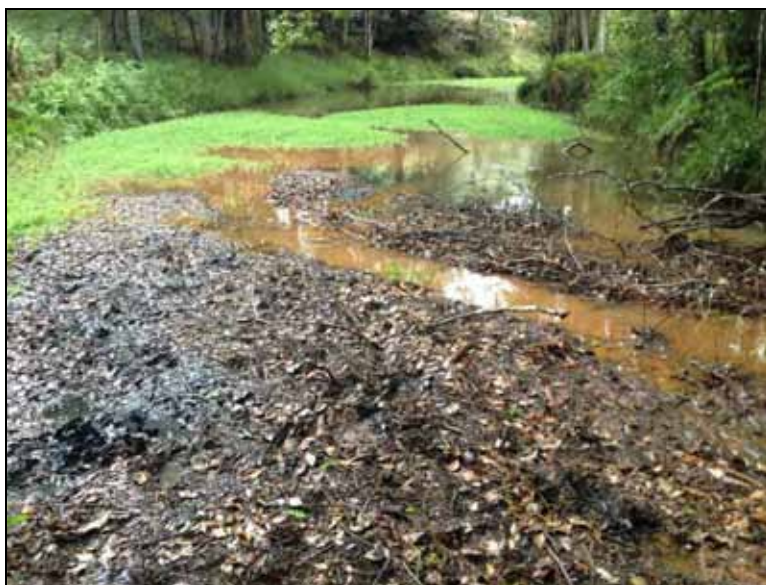
Plate 3: Pond located above culverts at Harrys Road – view looking downstream towards culverts (note dominance of the aquatic weed Parrots Feather Myriophyllum aquaticum )
