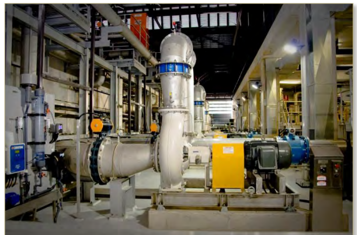
Bray Park Water Treatment Plant.
