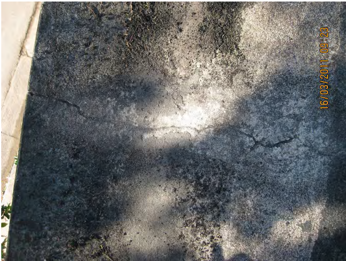
Figure 8 – Cracks over soffit water damage
