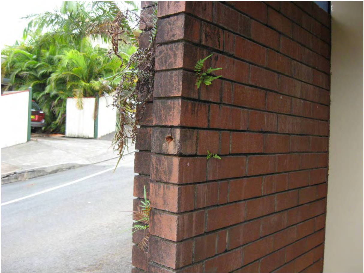
Figure 11 – Bolt Damage splitting brick
