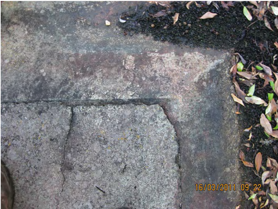
Figure 9 – Cantilever cracking and gutter debris
