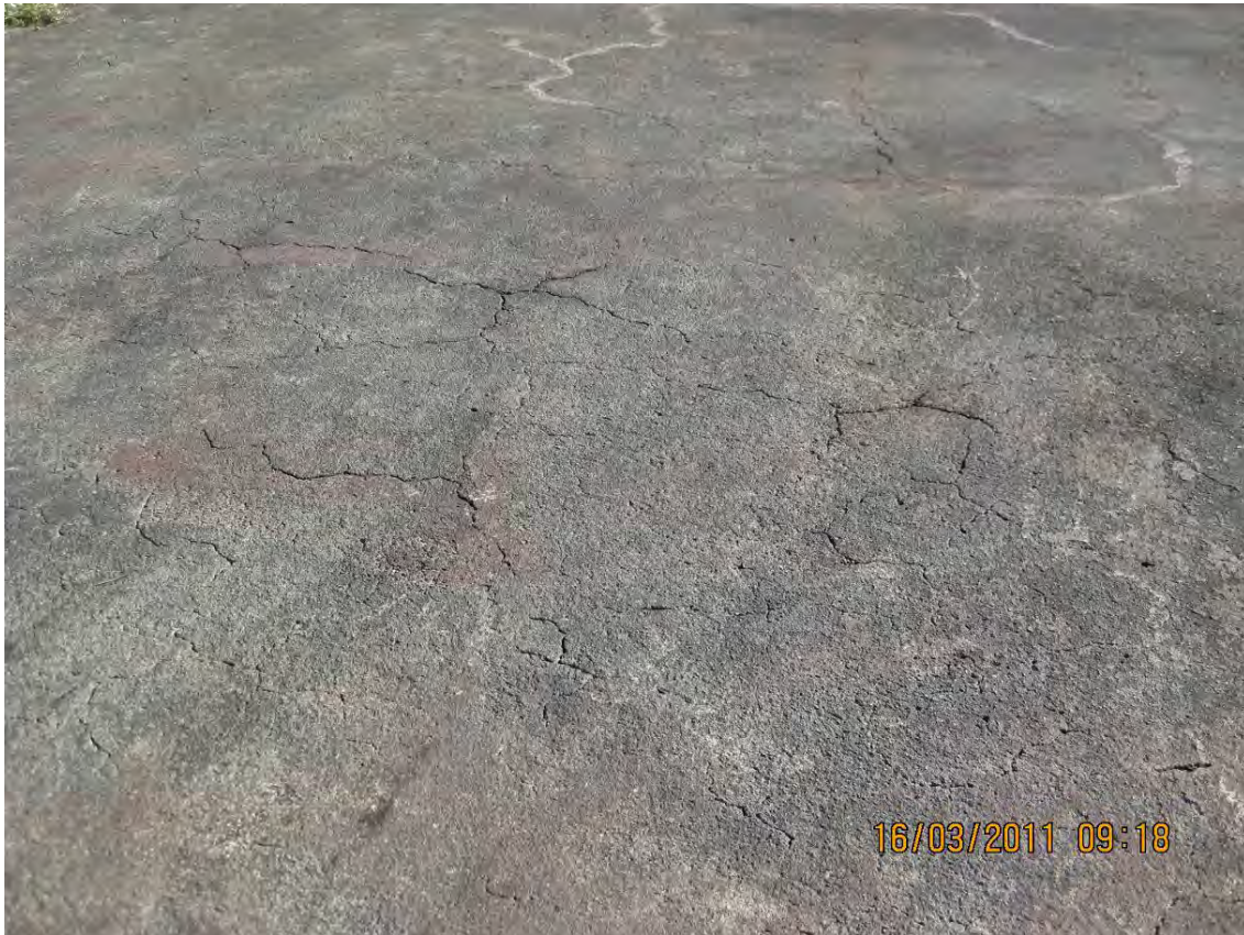
Figure 7 – Roof Slab Cracks
