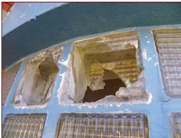
Figure 3.16: Broken glass bricks on the south elevation.
