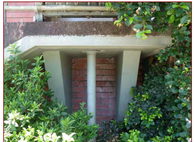
Figure 3.13: The stair supports, with later steel support. Water damage can be seen on the bricks behind.
