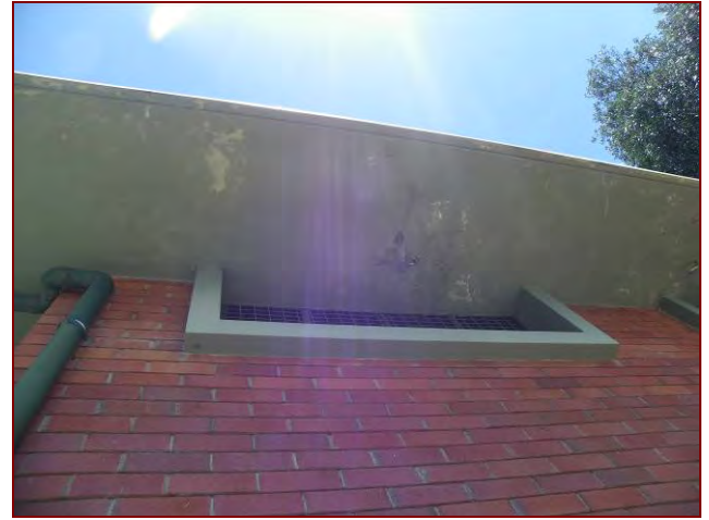
Figure 3.11: Cracking and water damage under the eaves of the east elevation.
