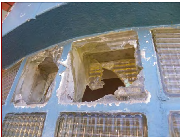
Figure 3.16: Broken glass bricks on the south elevation.
