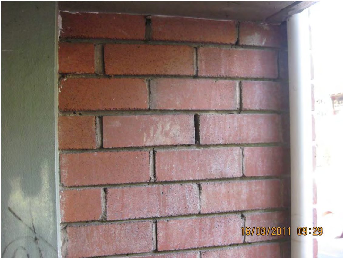
Figure 3 – Northern wall crack
