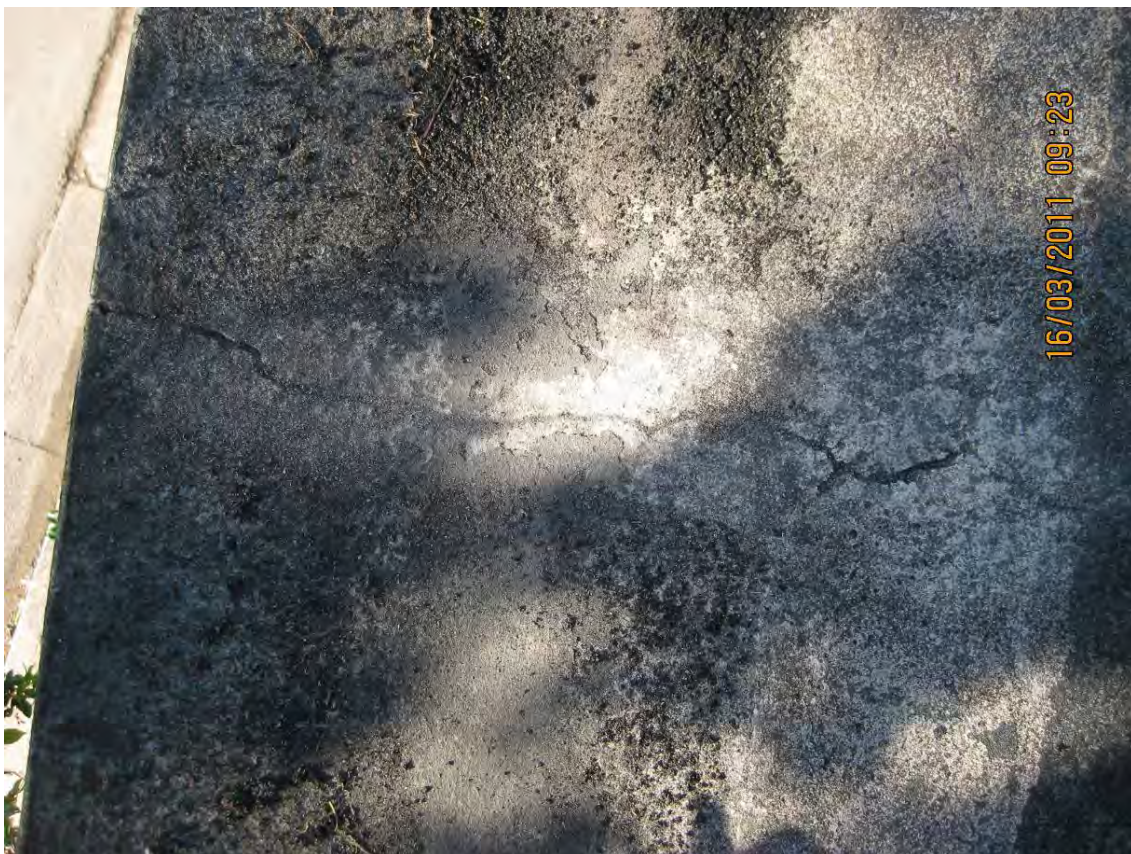
Figure 8 – Cracks over soffit water damage
