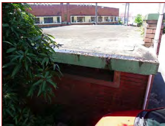
Figure 3.9: North elevation showing cracking of roof slab.
