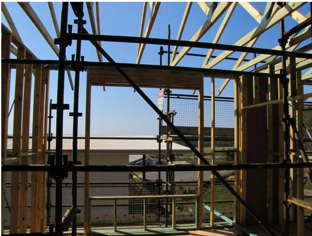
Photo 2 (above) is taken from the objector's home presently under construction and indicates that at this section of the house the horizon is not visible over the roof of the house at the subject property.
