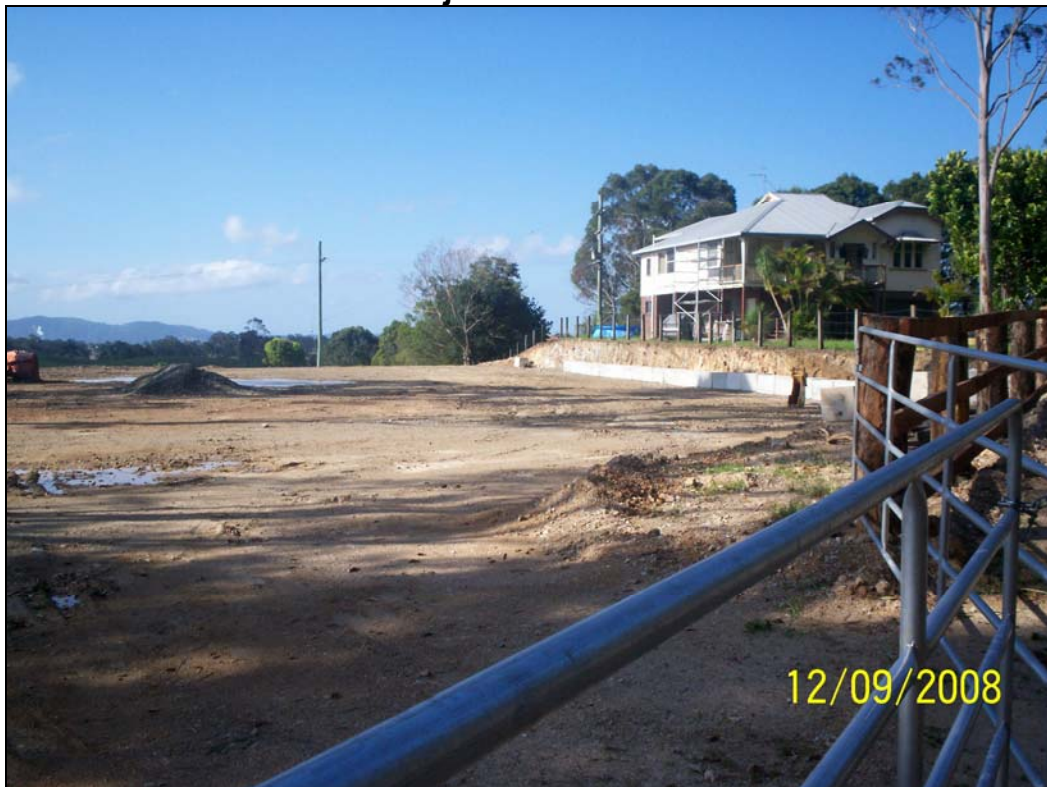
The subject site after unauthorised works
