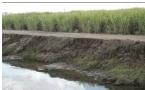
Example of cane drain erosion
