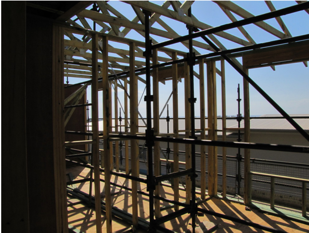
Photo 3 (above) is taken from the objector's home presently under construction and indicates that at this section of the house the horizon is visible over the roof of the house at the subject property (as the middle of the subject properties roof is lowered).
