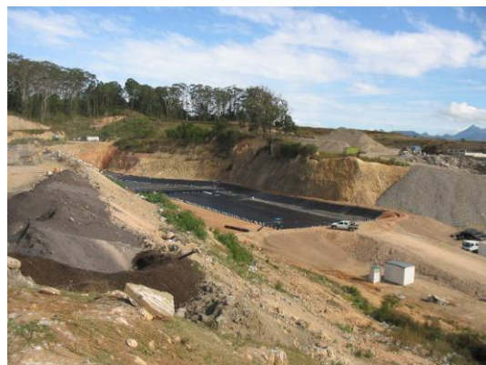
Putrescible landfill cell – stage 3 - constructed at Stotts Creek to accommodate approximately 18 months of landfill waste
