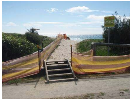
Picture. 2 – Temporary steps provided over sand pumping pipe. No handrails provided for steps.
