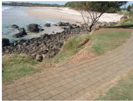
Picture. 5 – Edge drop off noted along Tweed Terrace.
