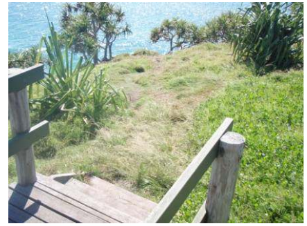
Picture. 3 – Steep stairs and drop off at top of Norries Head lookout. No barrier fencing provided at time of assessment.
