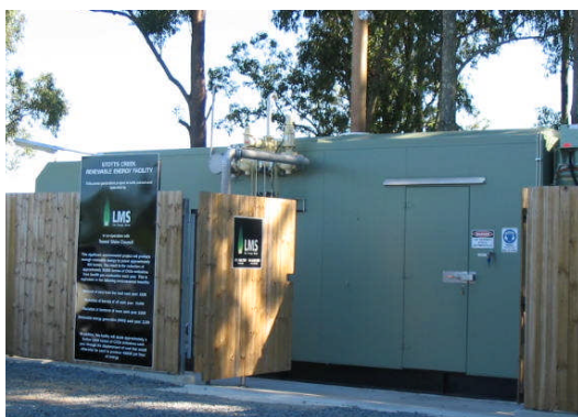
Landfill gas management at Stotts Island. The methane gas extraction system feeds electricity into the power grid
