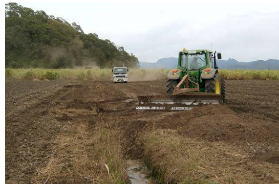
Filling of excess drains to reduce the export of acidity from acid sulfate soils
