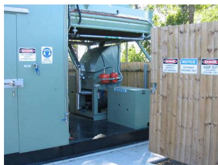
Landfill gas management at Stotts Island
