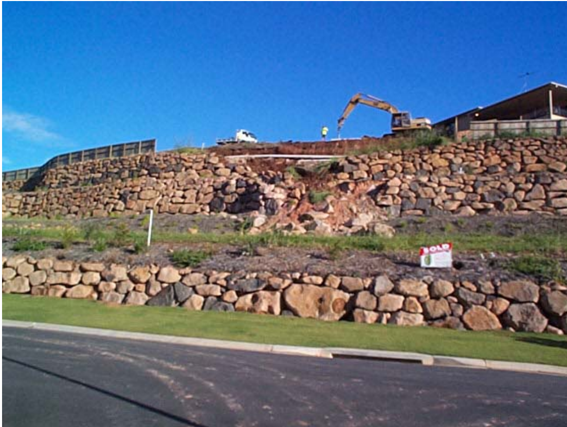
Fig 1. Retaining Wall Failure Bulwarra Place, Bilambil Heights
