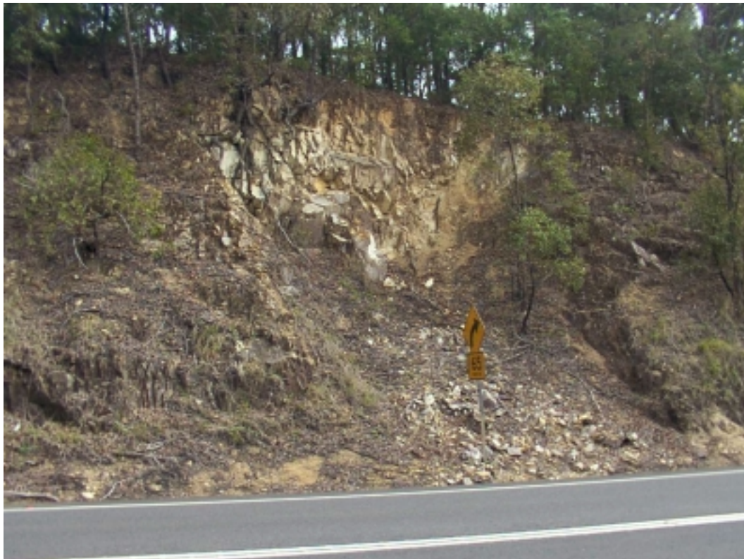
Photograph 1. Overhanging rock section at distance 120m
