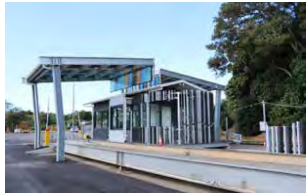
The new upgrades at the Resource Recovery Centre, including the weighbridge, will make it easier and safer for residents to dispose of their waste.
