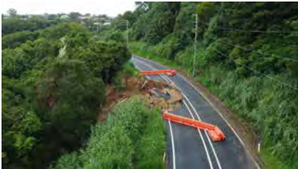
Geotechnical testing was conducted on the main landslide at Scenic Drive in the months after the flood to determine the best way forward to repair the road.
