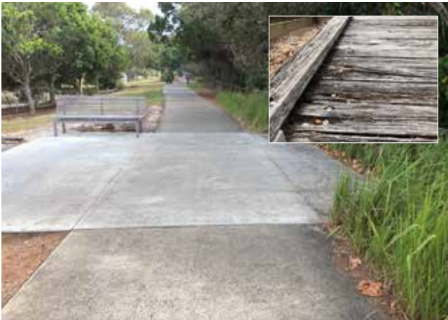
Old, rotting timber (inset) on shared-user paths was repaired between July 2016 and mid-2021.
