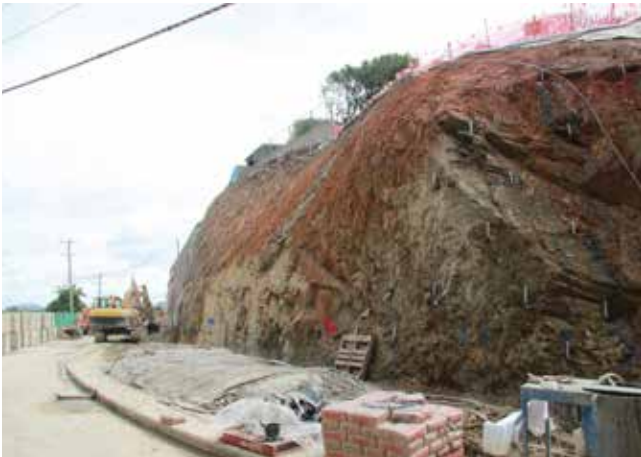
The cliff face on Tumbulgum Road prior to stabilisation.
