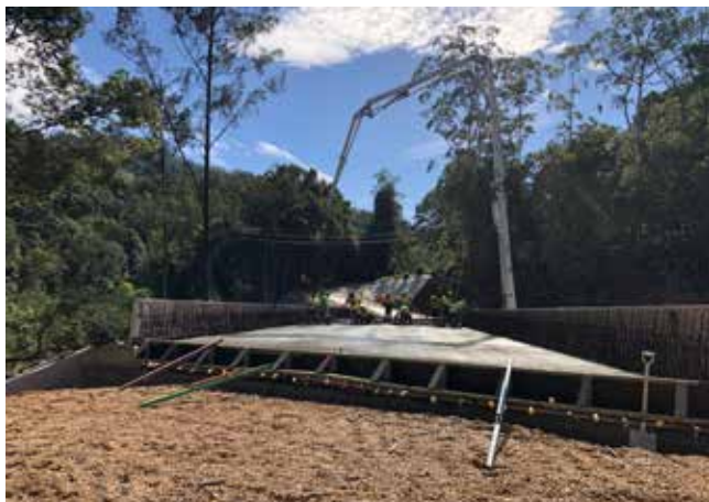
Byrill Creek Bridge was one of many repairs and rebuilds following the March 2017 floods.
