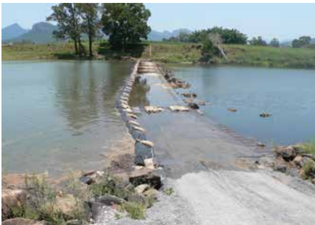
A hinged barrier at Bray park Weir will help mitigate the risk of saltwater contamination of the Tweed District Water Supply.
