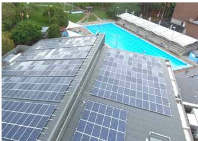
The 486-panel array (165kW) at the TRAC Murwillumbah.
