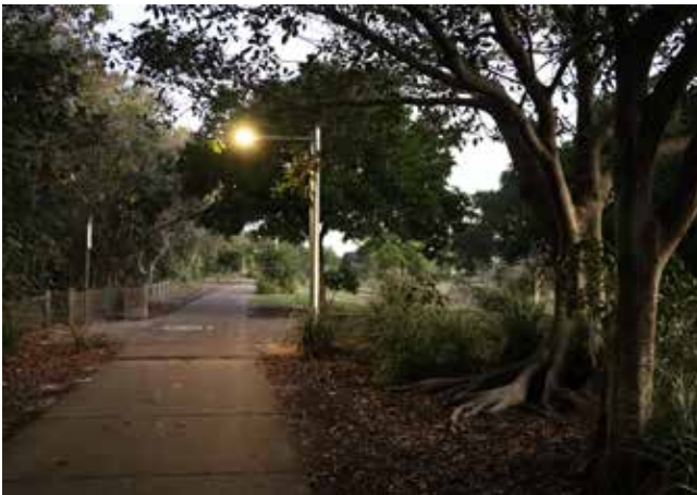
3.5 kilometres of new overhead cycleway lighting were installed between Salt and Casuarina.
