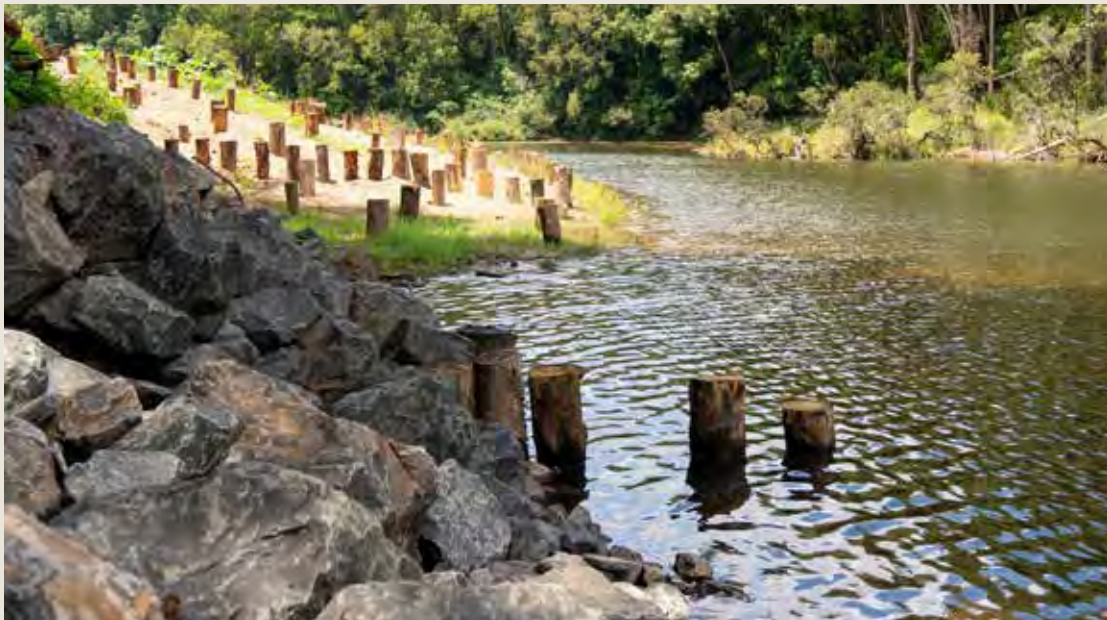
The project involved installing rock revetment along unprotected sections of riverbank and around 1,700 hardwood logs were driven into the riverbed in rows, designed to capture natural sand and gravel to rebuild riverbed levels.
