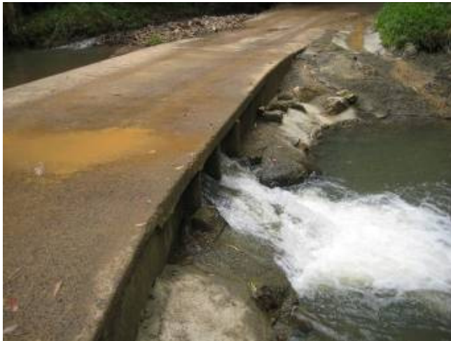
Figure 13.14. Culvert bridge fish passage barrier, upper Bilambil Creek (Site 9).
