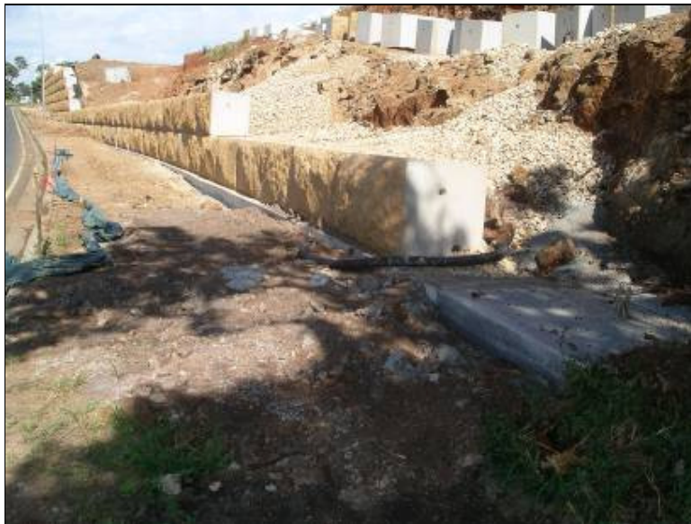
Figure 13.13. Poorly maintained erosion and sediment control devices within the Terranora Broadwater catchment
