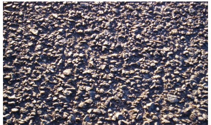
Aged surface condition if asphalt is not treated. Further deterioration will result in potholes and failures.
